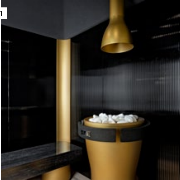
1- The ceiling-mounted outlet releases a water mist onto the hot oven stones.
